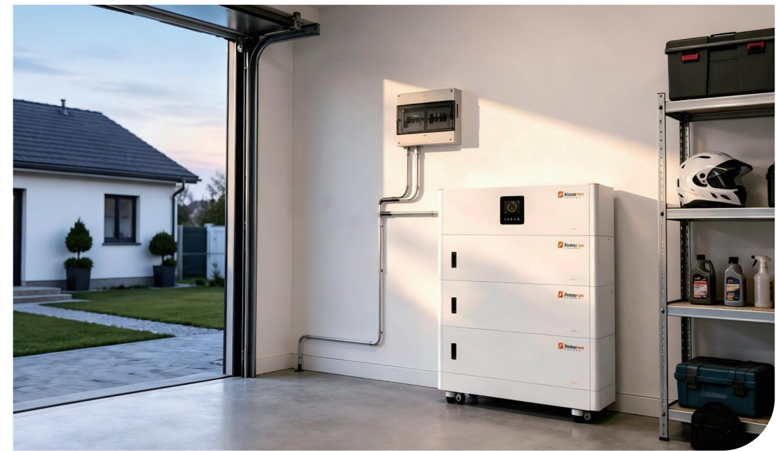
Romania | Residential Backup Power System 5.5kw/15kwh | Off-Grid | Self-Sufficient | Indoor Installation
